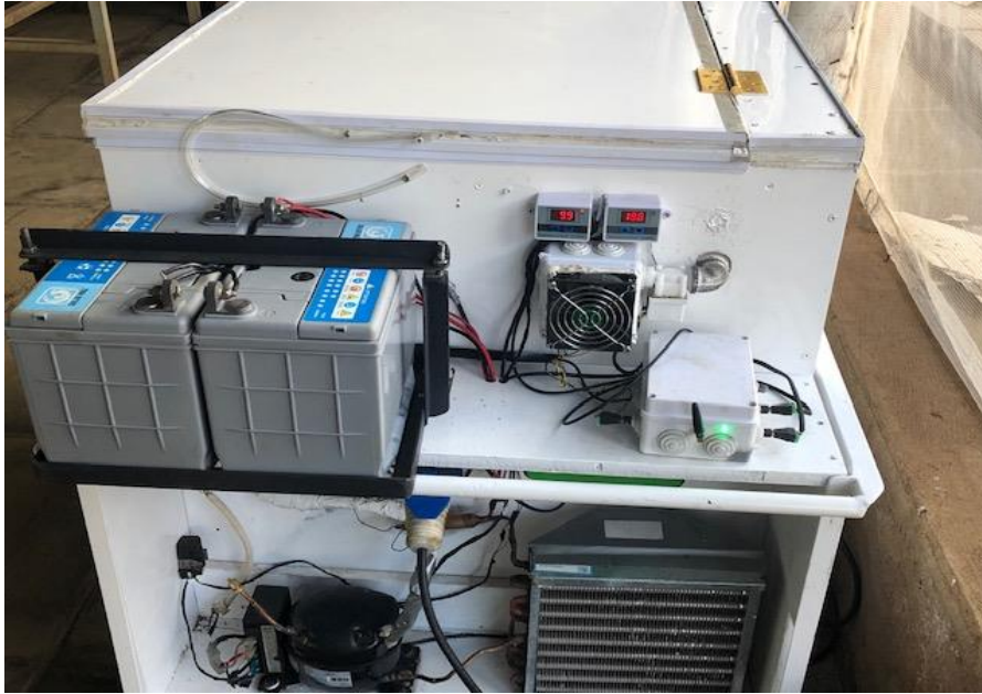
Figure 6. 5- Cold store with solar-powered vapor compression refrigeration system.
