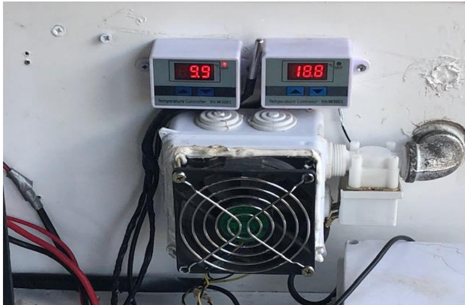
Figure 6.3– Temperature display panel for cold chamber and produce chamber
