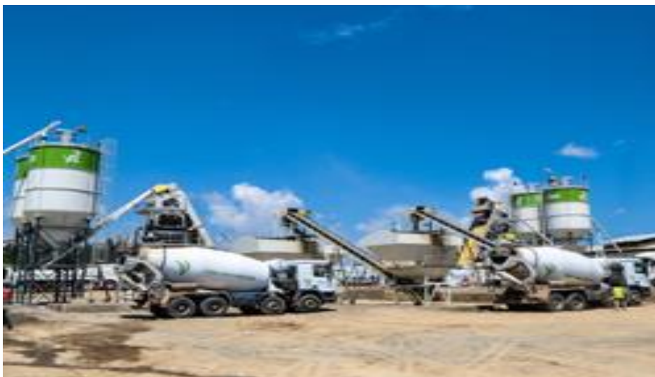
Plate 2.1: Modern Concrete production plant (by large contractors and suppliers) Source: Kajima Construction company site, Debre markos road project Ethiopia 1999.
