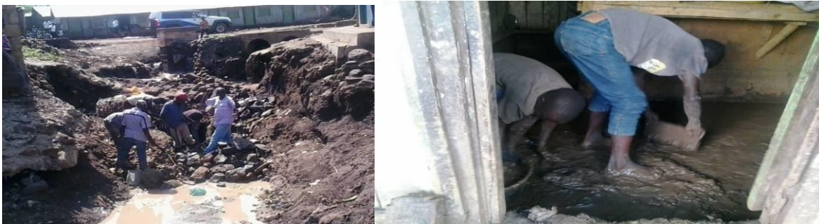
Plate 6.3: a) Left: Residents repairing gabions along Merille River; b) Right: Residents scooping mud from affected houses along Merille River.
