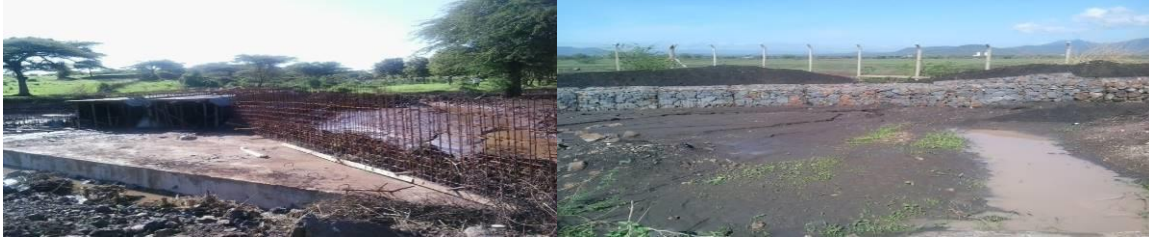
a) Bridge being constructed along Merille River b) Gabions put up as diversion of floods at the airport
