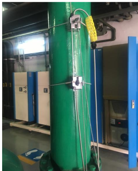
Figure 3.2: Flexim Ultrasonic Flow meter clamped on water line to cooling tower.
