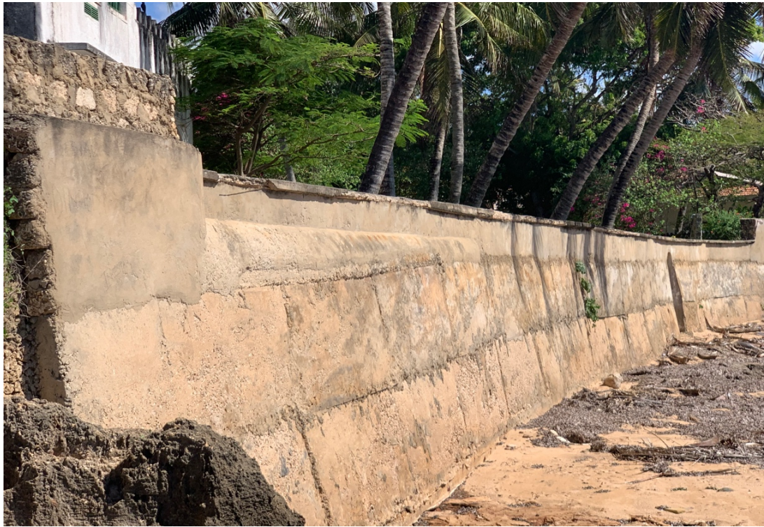
Figure 5.8: Illegal Wall constructed along the beach
