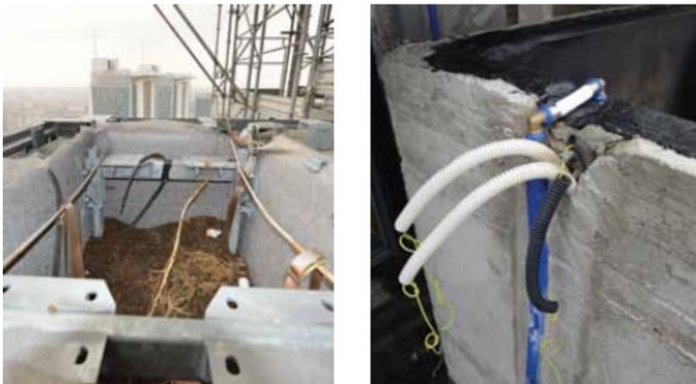
Figure 2.22: Bosco Verticale's plant container layer membrane and plant container's drainage system Source: (Giacomello, 2015)
