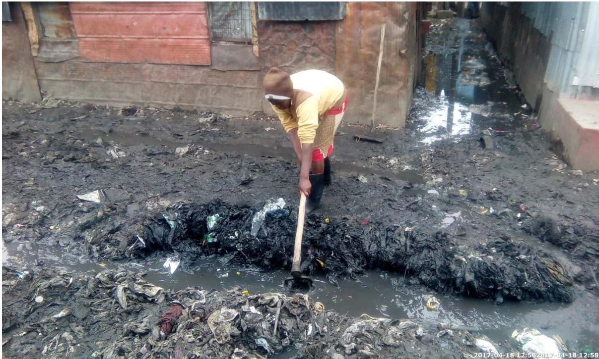
Figure 4-9: Mukuru kwa Ruben resident digging and clearing a trench near her house (Author, 18/04/2017)
