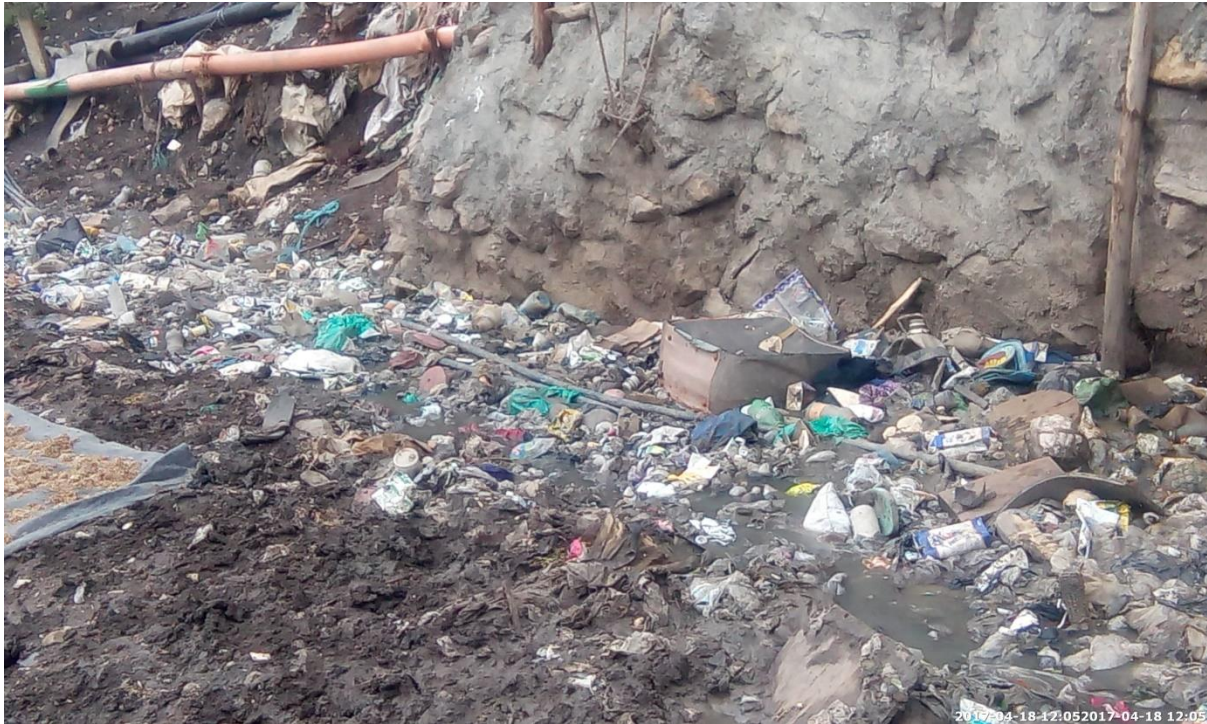
Figure 4-5: Potable water pipes passing through a waste leachate in Mukuru kwa Reuben (Author, 04/18/2017)
