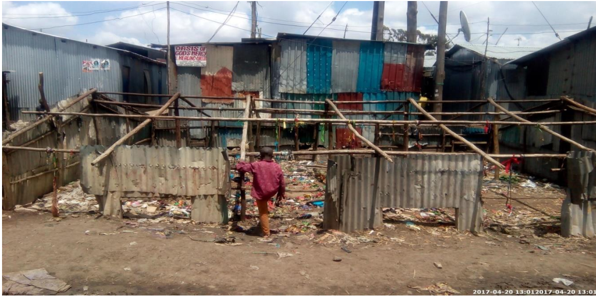
Figure 4-7: One of the house structures in Mukuru kwa Ruben which sunk (Author, 20/04/2017)
