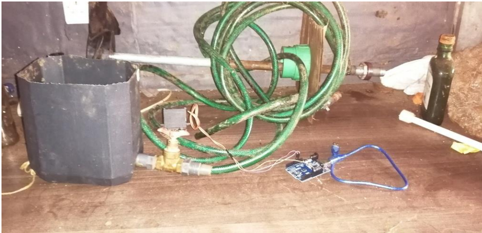
Figure 3.24: Arduino controlled servo for warm water circulation
