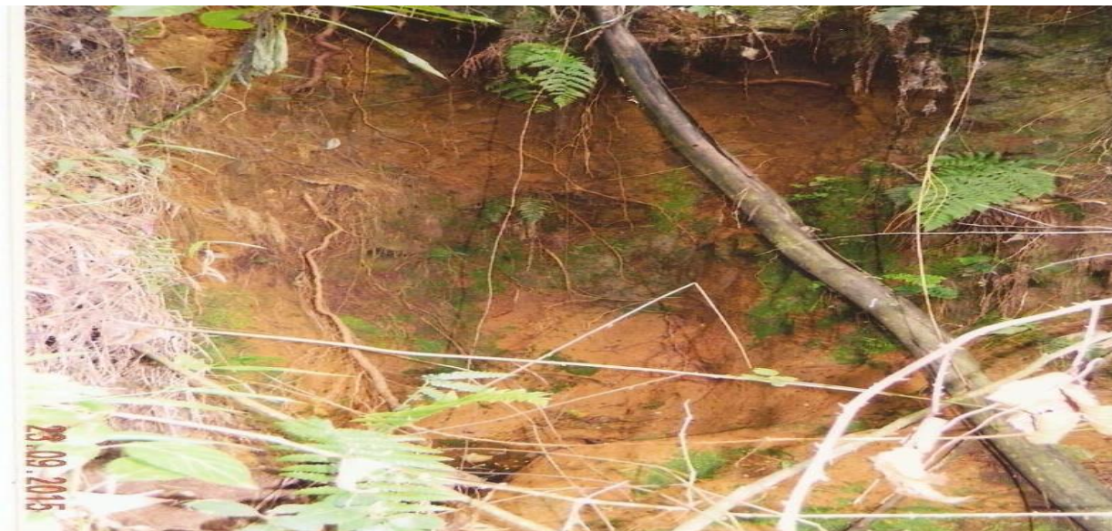
Plate 10: Section of Land affected by Landslide
