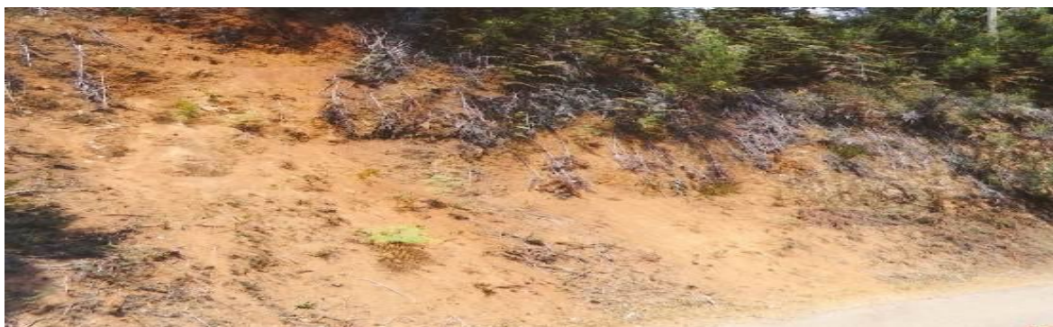
Plate 12: Eroded Roadside due to Heavy Rainfall
