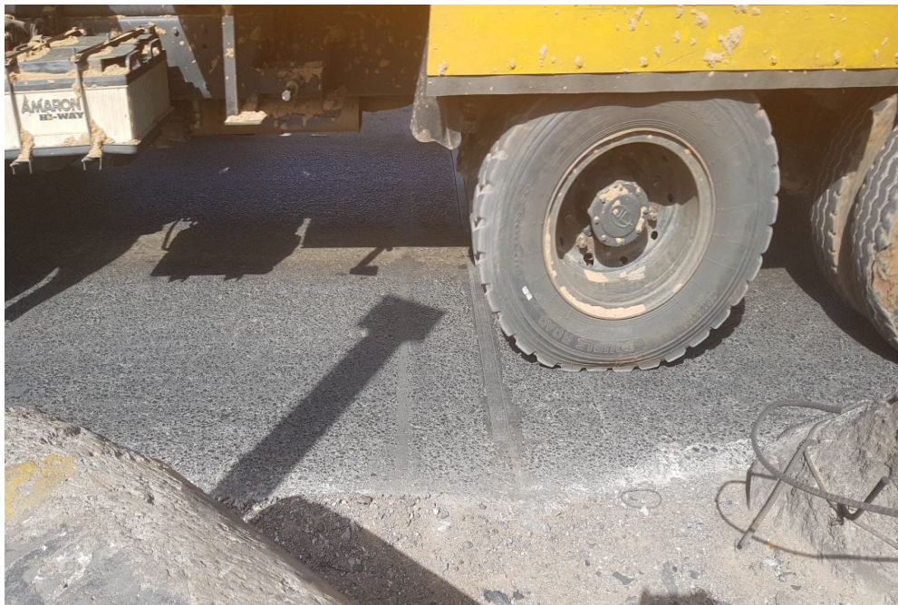
Plate 1.8 Damaged gravel surface at the weighbridge location
