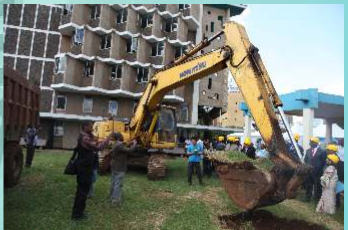
The ground-breaking ceremony for the construction of the University of Nairobi Towers on 17 May 2013 presided over by the Chancellor Dr. Joseph Barrage Wanjui.
