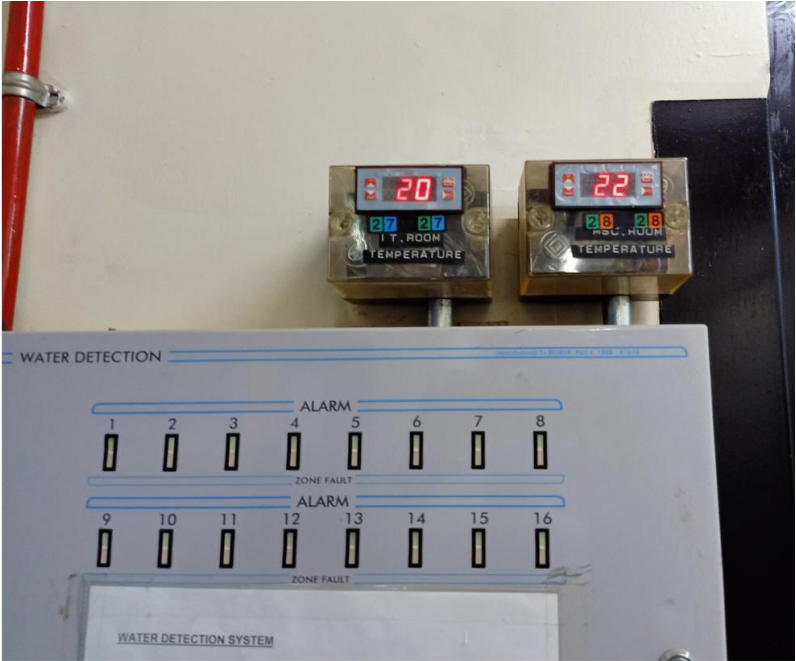
Figure 29 PSK001 data centre door LCD displays showing temp readings
