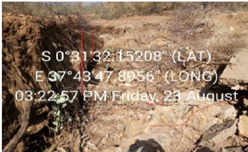
Figure 5.2: Retreating gully head by failures in the upper-segment region
