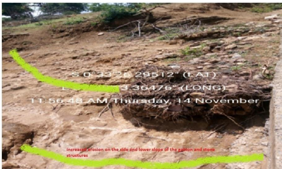
Figure 5.26: Excessive erosion downslope over rehabilitation structure
