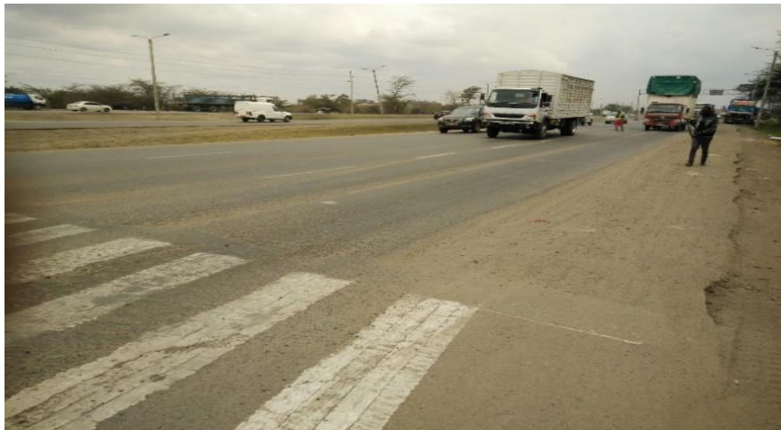
Plate 4-5: Plate showing a section that has undergone edge spalling
