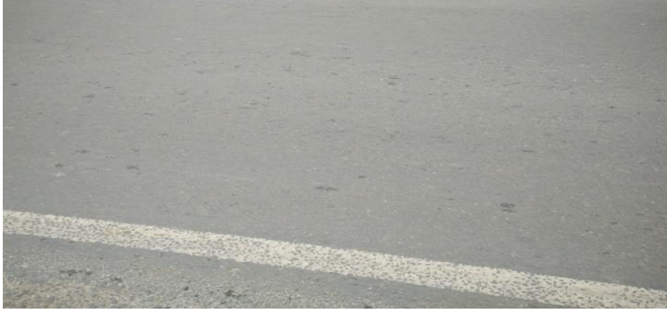
Plate 4-6: Bleeding of the asphaltic binder
