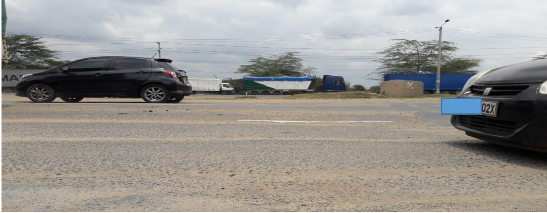
Plate 4-2: Excessive rutting on pavement surfacing
