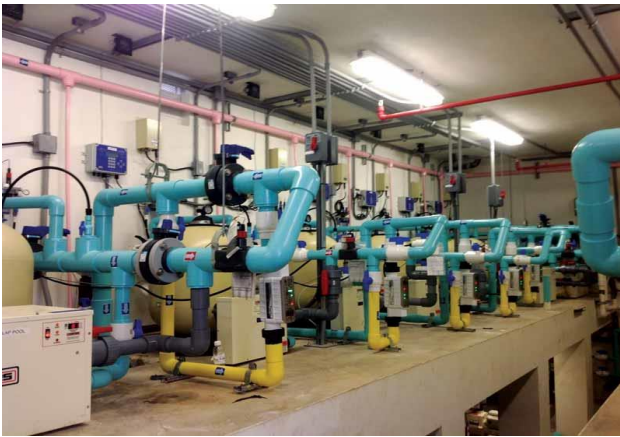
Figure 2.18: Perspective of a pump room Source: https://www.poolspmarketing.com/trade/features/designing-for-functional-operations-practical-considerations-for-commercial-pump-rooms/
