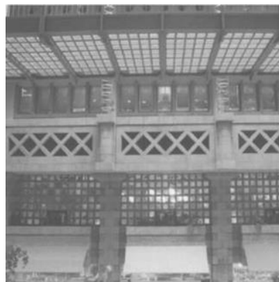
Figure 2.74: Fresh air intakes via the cross chevron screens with a parking area below and the skywalk above Source: https://www.researchgate.net/figure/Eastgate-Center-Harare
