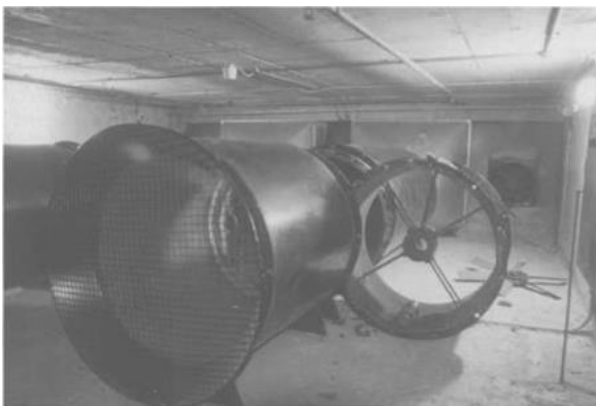
Figure 2.72: Typical fan room with the day fan housed in the back wall (right) and the night fan out of its circular duct housing for repair Source: https://www.researchgate.net/figure/Eastgate-Center-Harare
