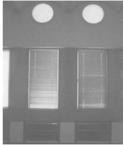
Figure 2.73: Air supply grilles under the perimeter windows. The grille on the left incorporates a small electric heater Source: https://www.researchgate.net/figure/Eastgate-Center-Harare
