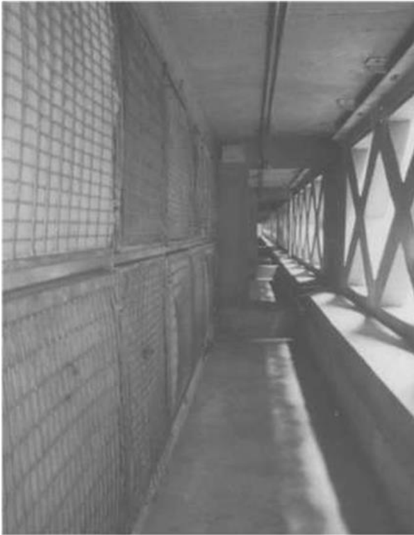
Figure 2.71: Filter bank between the fresh air inlet from the atrium (right) and the fan room (left, on the other side of the filters) Source: https://www.researchgate.net/figure/Eastgate-Center-Harare
