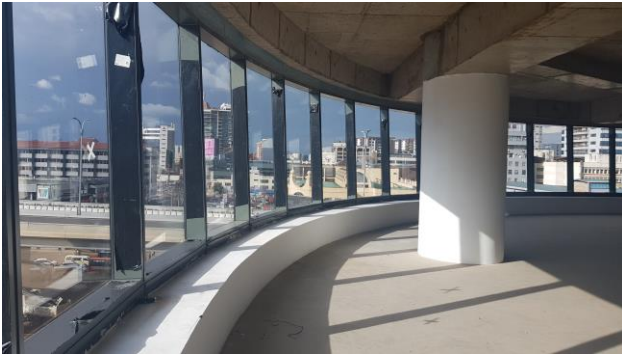
Figure 6.11: Fixed window panes in a lettable office at One Africa Place Source: Author
