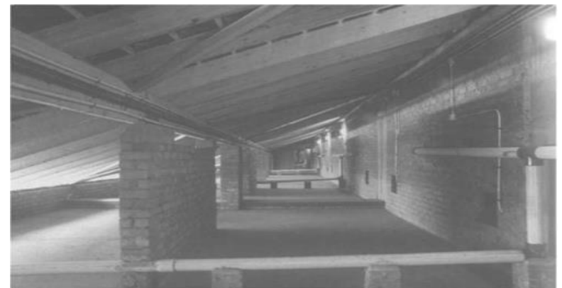
Figure 2.76: Ventilated loft space above the office floors. The square grilles on the right hand wall are the exhausts from the toilets. The foreground piping is part of the drainage system from the chimneys Source: https://www.researchgate.net/figure/Eastgate-Center-Harare
