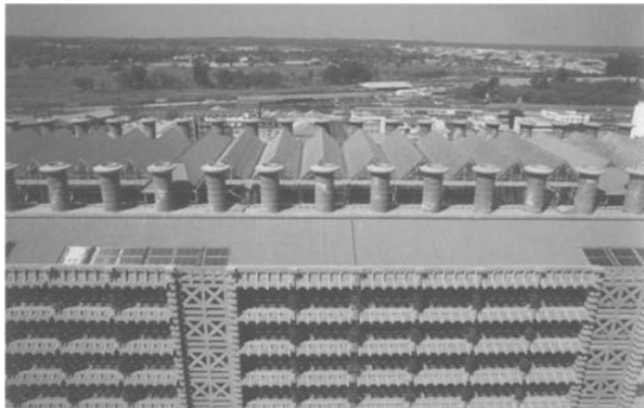
Figure 2.78: Perspective of the roof showing the chimney and canopy layout Source: https://www.researchgate.net/figure/Eastgate-Center-Harare
