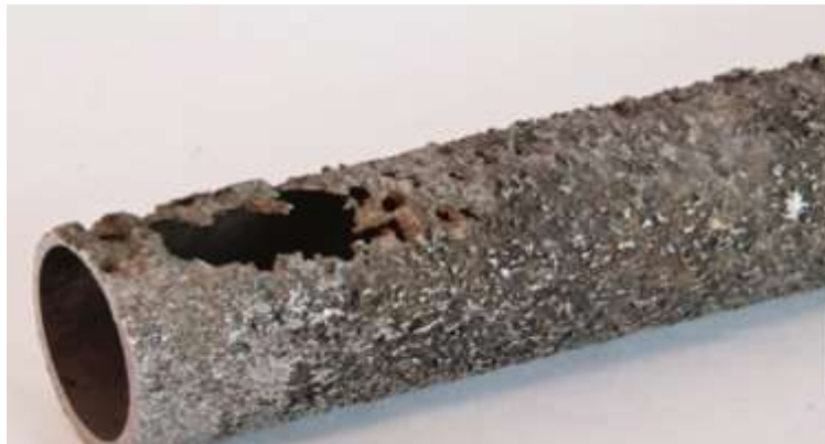
Figure 1.1: Rusted material (Evans and Taylor, 1972)
