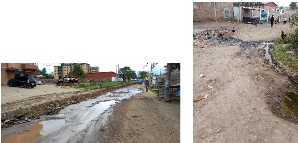
Figure 34: Kwa Muthaura Road in poor condition (left) condition of some of the roads connecting Kware Market (right)
