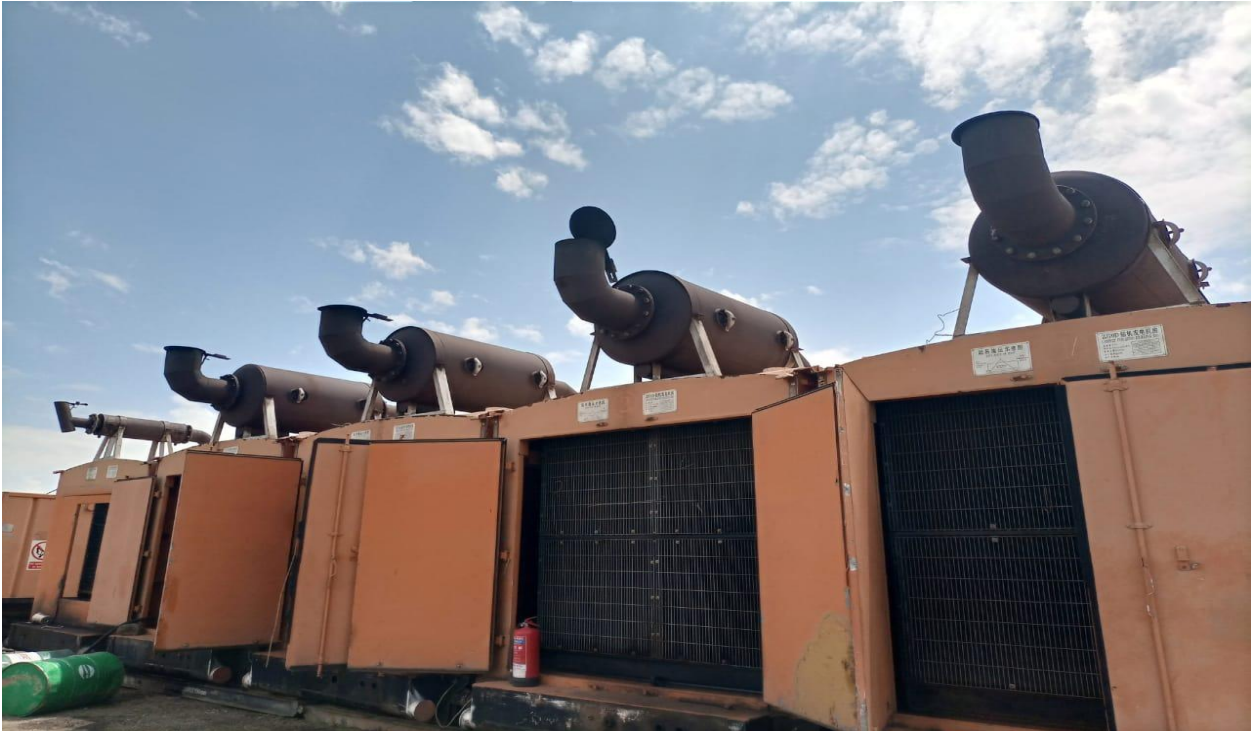
Plate 4. 9: Excessive Noise from Generators and are also Hot Surfaces
