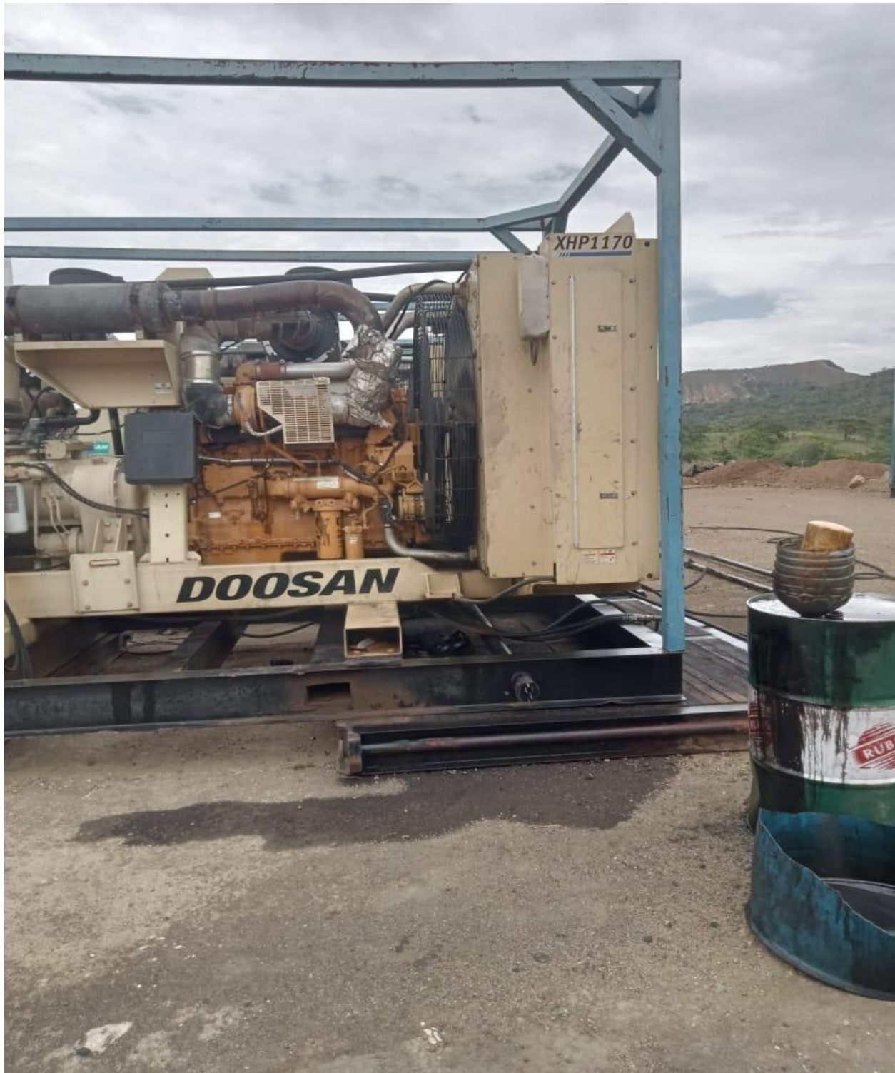
Plate 4. 5: Exposed Compressor Propeller
