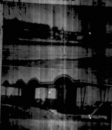
Work in progress on the drive-in cinema. Drivers enter the cinema from the top left corner.
