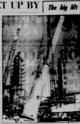
These cranes lifted this 60-ton, 190-ft long "blow down" stack into position at the Brown Petroleum Co. Kansas City refinery in Western Australia, near Perth, in under 20 minutes. The stack is the highest vertical structure in the refinery's new $42,000,000 capacity re-refining plant.
