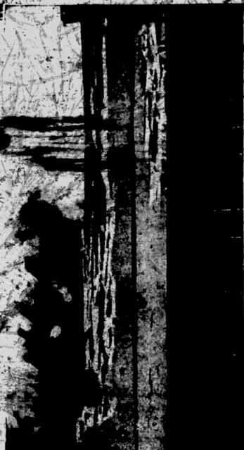
Due to lack of protection, the destruction caused by White Ants was so great in this structure as to render it useless in an incredibly short time.
