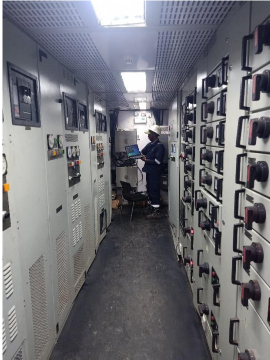
Appendix Figure 1 - 1: The SCR Room data collection
