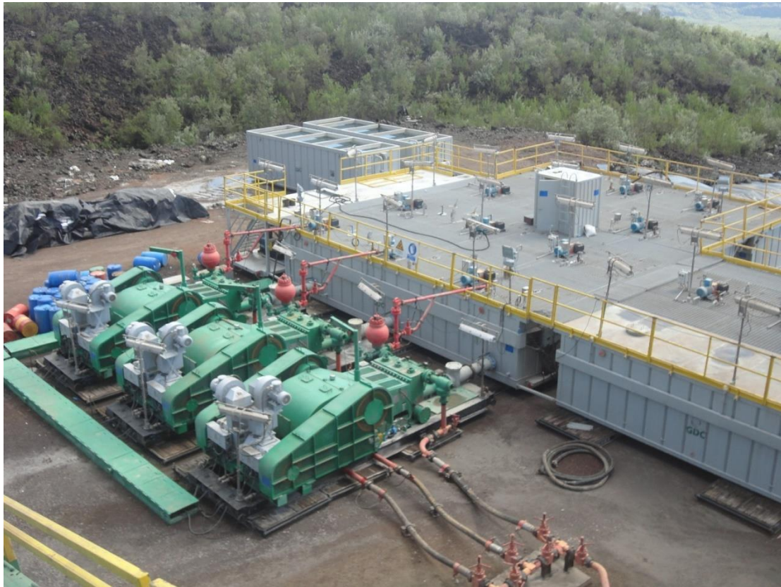
Figure 2 - 10: Triplex mud pumps [Menengai]
