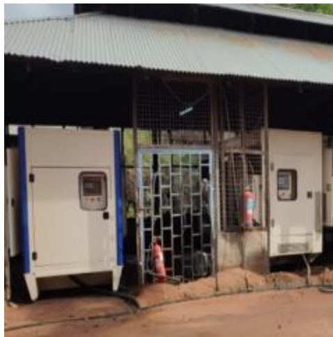
2 x 550kVA Generators
