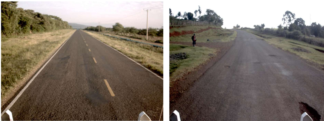
Figure 4-1: Minor distress (bleeding) and lack of drainage system on Kampi ya Moto-Kamwosor Road (source from the field)
