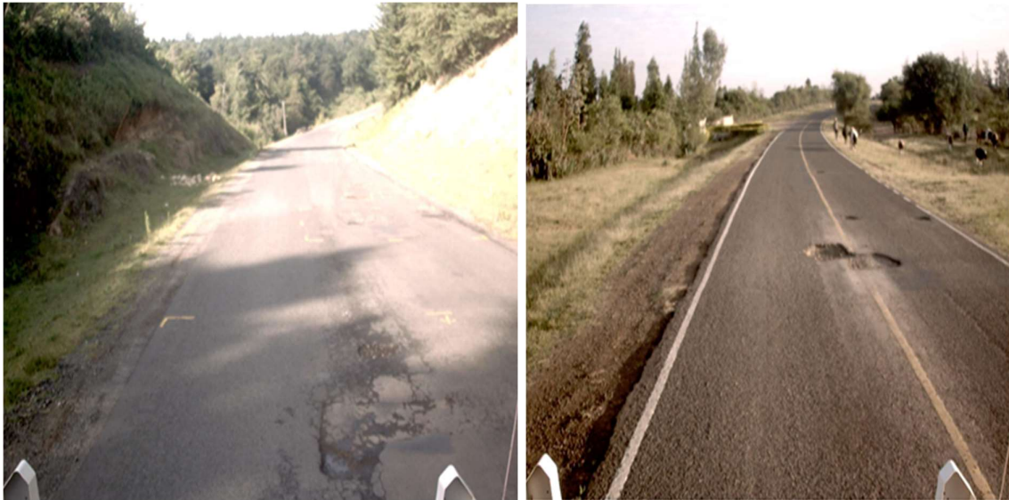
Figure 4-3: Major distress on Kampi ya Moto - Kamwosor Road (source from the field)
