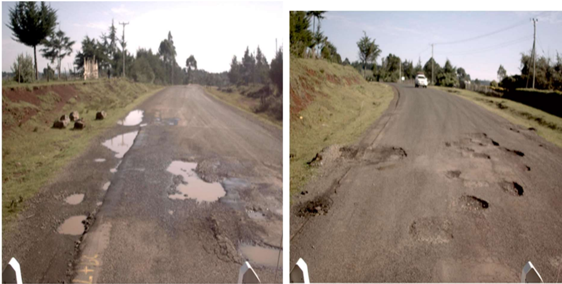
Figure 4-2: Major distress and lack of defined system. (source from the field)
