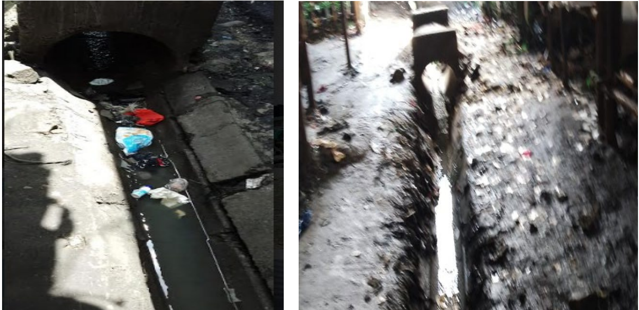
Picture 5 Liquid Waste Disposal System in Kamukunji Market, Source: (Camera photo 2024)
