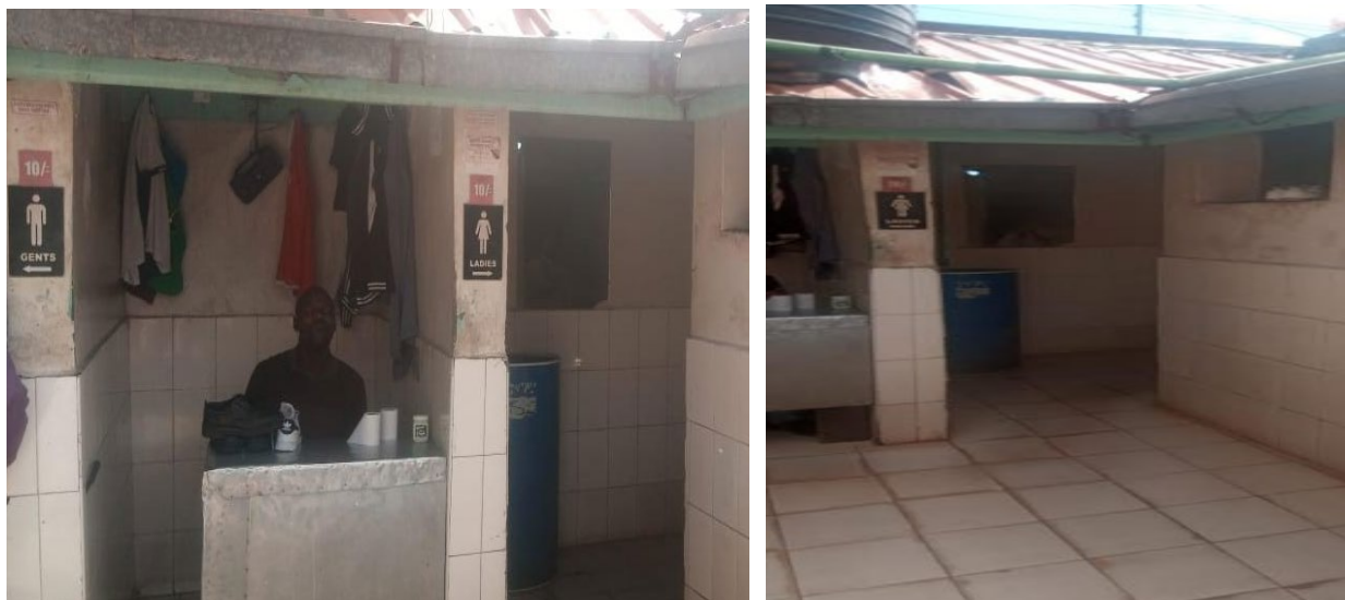
Picture 16 State of Public Toilet in Burma Market, Source: (Camera photo 2024)
