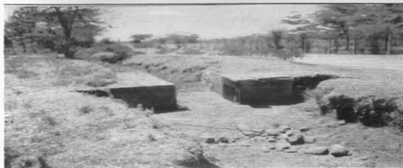
Plate 4.3: Intake of Matuu water supply at the canal. (Picture taken on 6/2/06)
