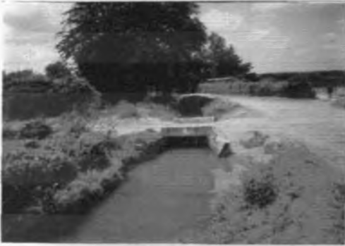
Plate 4.1. Breached canal embankment at Km 11
