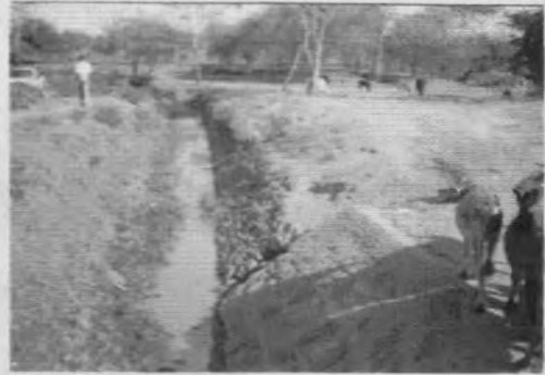
Plate 4.2: End of water flow in Yatta canal at Km 45 on 6/2/06
