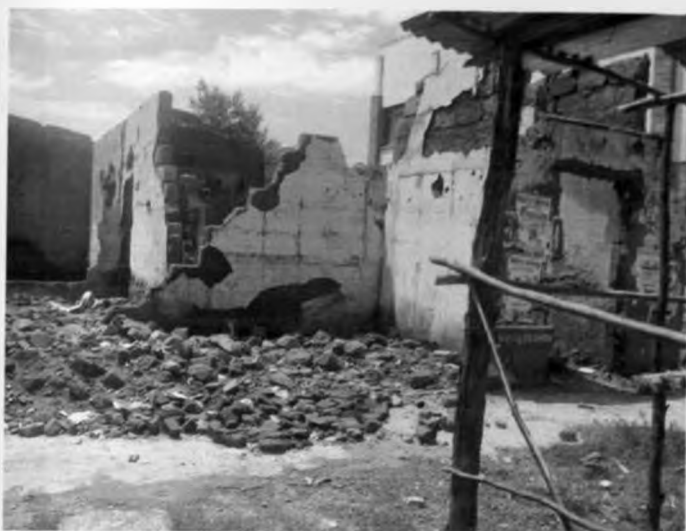
Illustration No. 4: Business premises in a state of disrepair in Kisumu City Photo by Researcher: October 24, 2008
