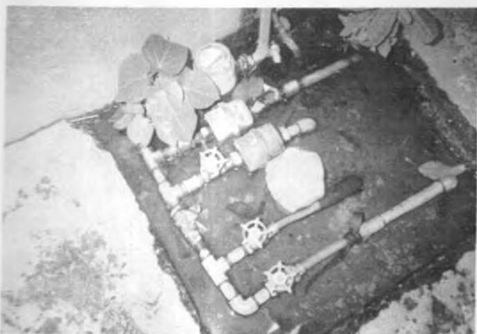
Photo X. Illegal water connections in Umoja II estate.
