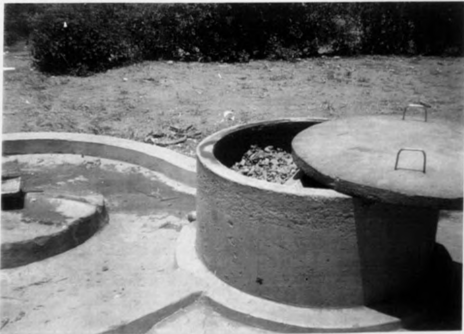
PLATE 12 Handiti iron removal plant (C-5462)
