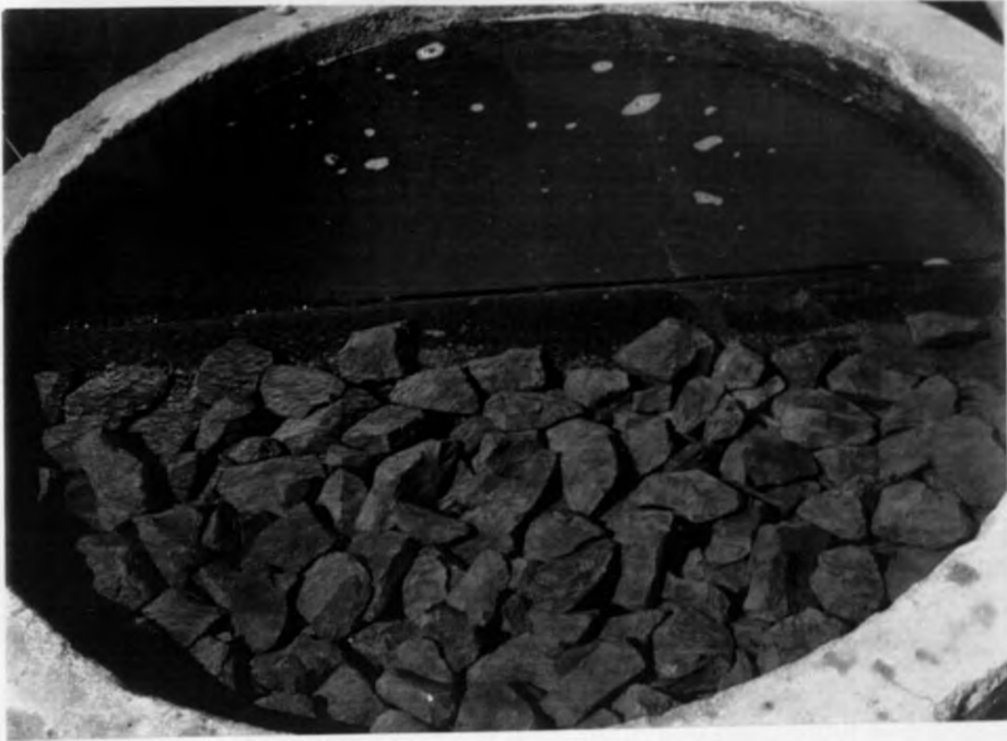
PLATE 1 Khayinga Plant immediately after backwashing
