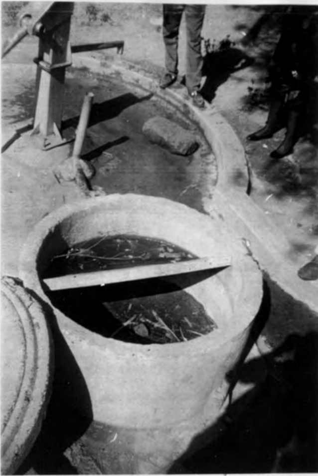
PLATE 11 Lutaso iron removal plant (C-5480)
