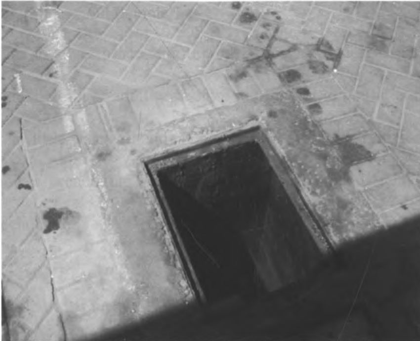
Fig. 12: Proper used oil handling system (spilled oil on the cabro works is simply washed off into the interceptor).
