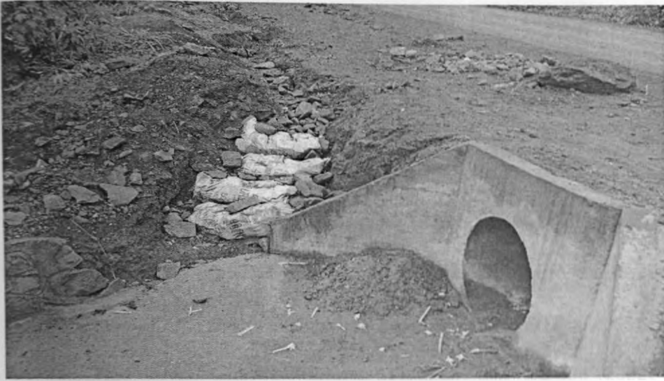
Plate 4.4: Badly maintained side drain along Mutunduri road next to Gully B discharging into cropped land.
