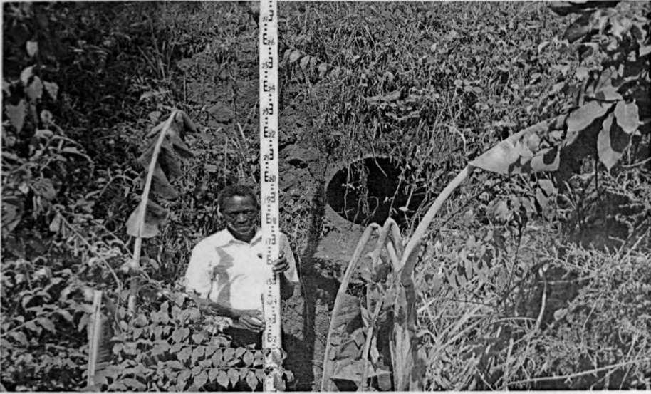
Plate 4.1: Culvert draining road runoff into Gully A
