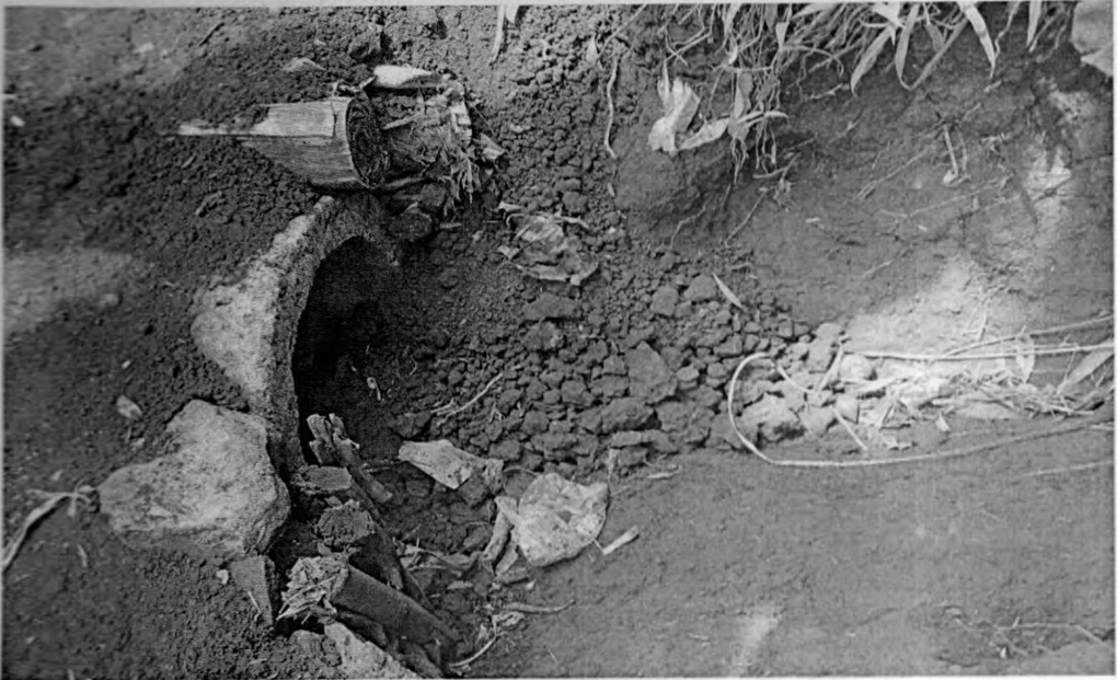
Plate A1: Blocked culvert near Gully A
