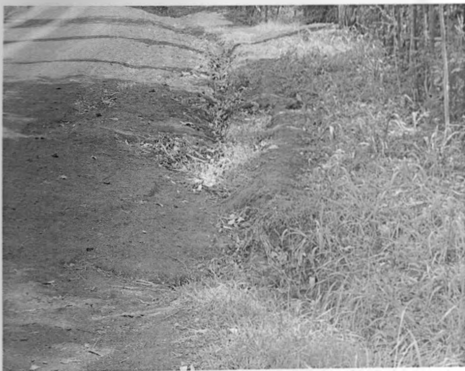
Plate 4.2: A badly maintained side and mitre drain that was draining into gully A
