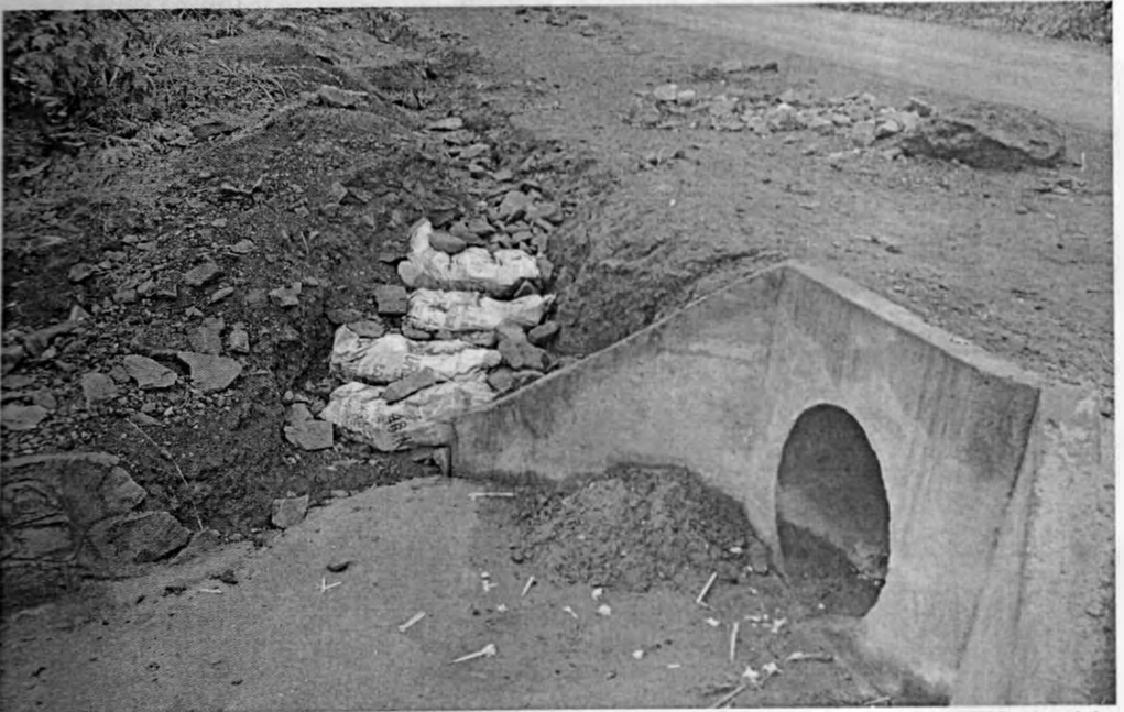
Plate A4: Controlling soil from entering the culvert using stones and bags filled with soil.
