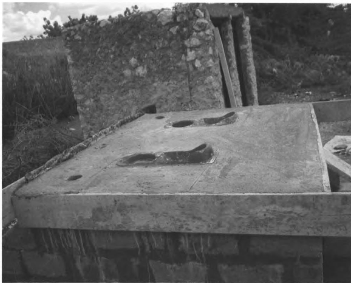
Plate 5.2: The substructure with the urine separation plates of a toilet in Wajir town under construction
