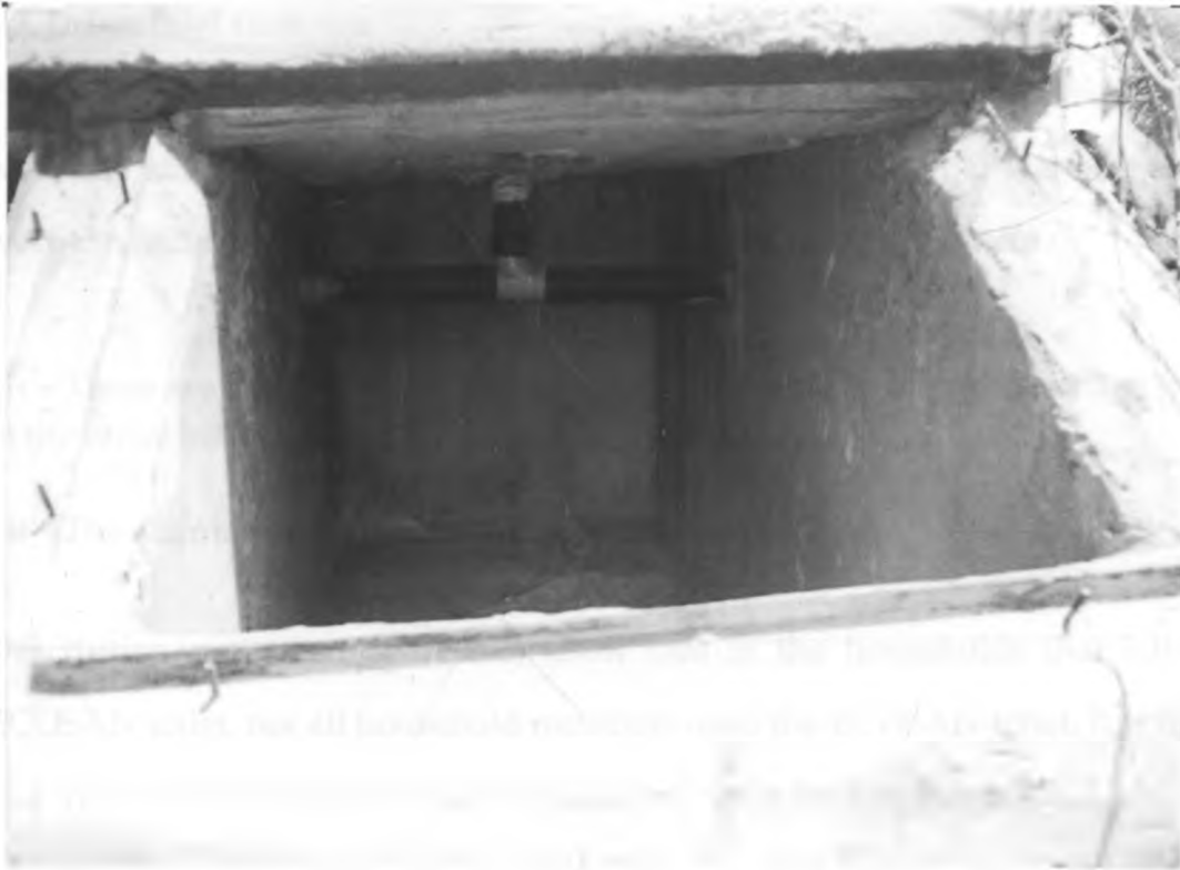
Plate 5.4: The inside of the chambers of an ECOSAN toilet in Wajir town
