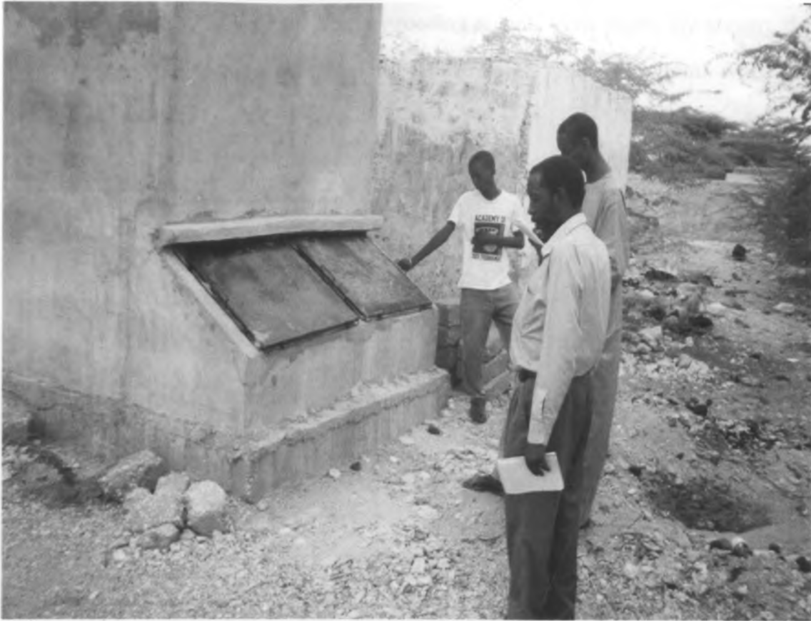
Plate 5.3: The back of an ECOSAN toilet in Wajir town, showing the double chambers.
