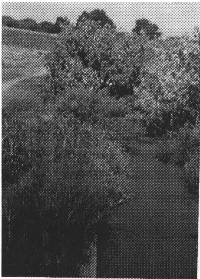
Plate 2 A lined distribution canal overgrown with weeds in block A: Nyanyadzi
