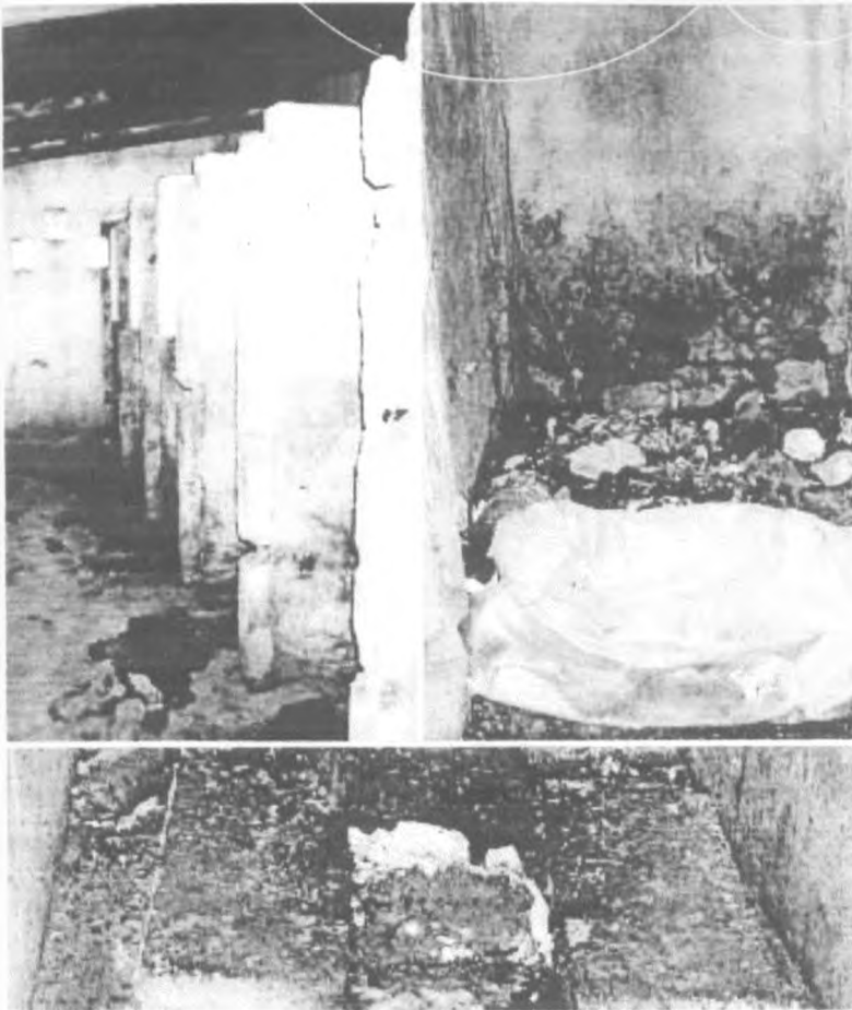
The dilapidated state of Nairobi's public toilets before rehabilitation
