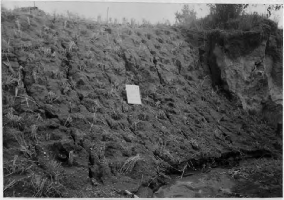
Plate 8. Part of the reshaped gully A wall showing rilling and soil washing at its toe region.
