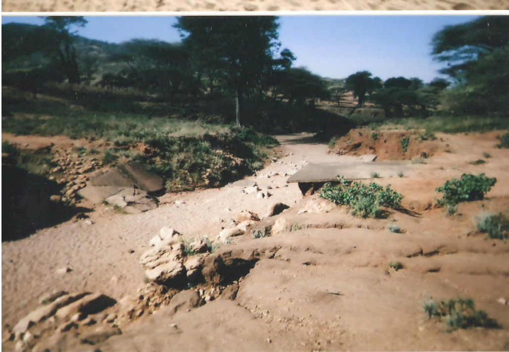
Photo 3. A landscape showing small gullies resulted from erosion after flash floods . In the middle is a dry riverbed and a damaged bridge that resulted from the floods.
