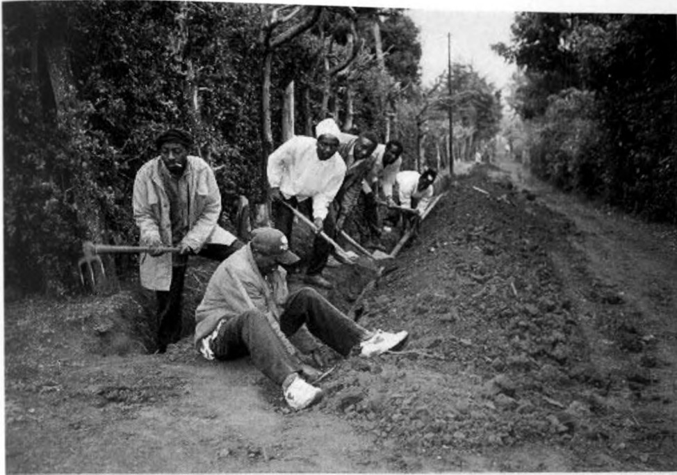
Plate 5.7: A picture showing work being carried out to rehabilitate the piping system of Gitangu Water Project, Kiambu District, Kenya, June 2000.
