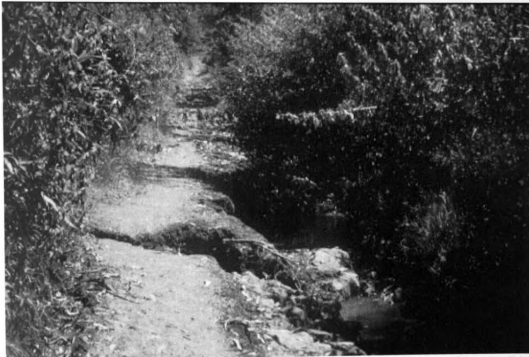
Plate 5.2: Photograph showing damaged access road to Kiawamagira ISS, Kiambu District, Kenya, October 1997.
