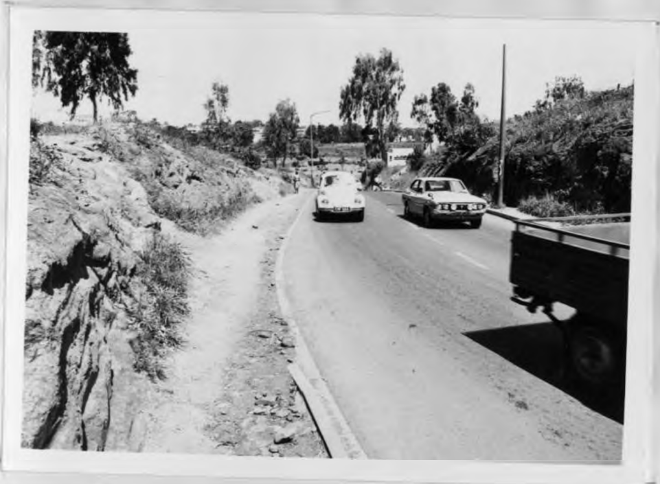
PLATE-19 Roads lacking proper pedestrian sidewalk(pavement)
