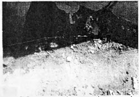
Plate 7: Burst water pipe exposed to contamination in the open drain (Source: Field Survey, 2006)
