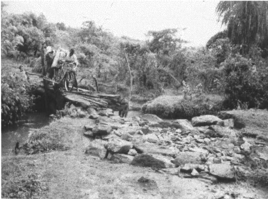
Plate 3.3: The state of the bridges in the study area
