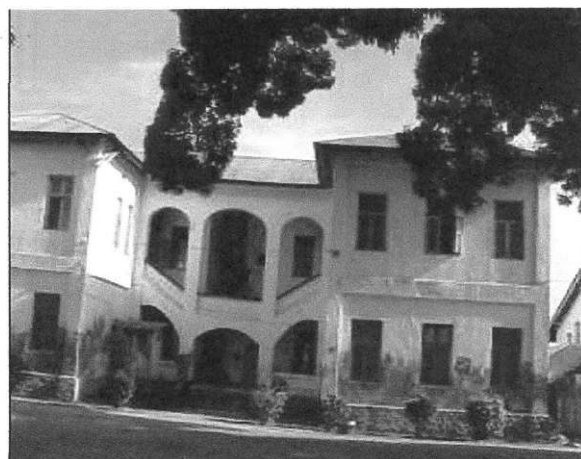
Plate 4.16: Peeling off of wall plaster and painting at lower part of building due to climatic condition effects, (health Building)
