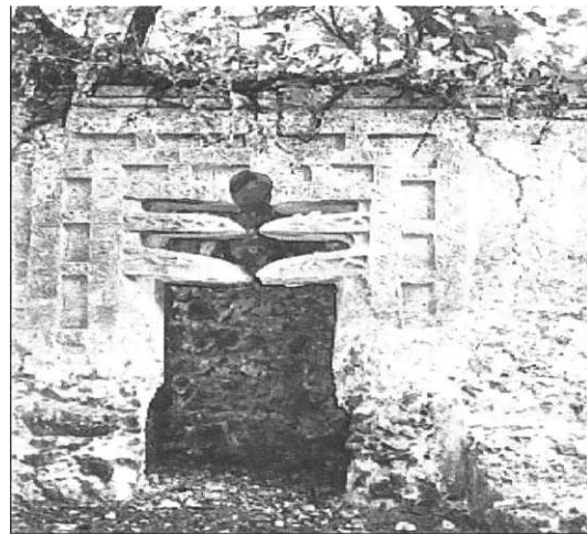
Plate 4.6: Cracks caused by plants at the Kwale
