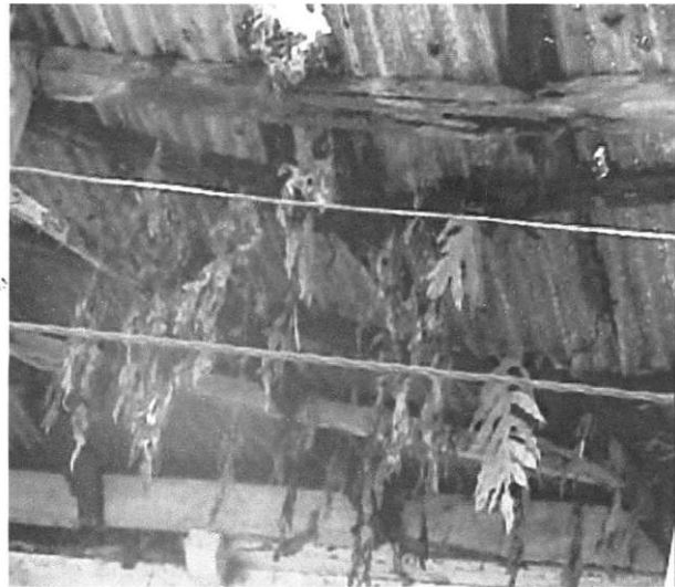
Plate 4. 8: highly corroded roof, Bohora building, Tanga
