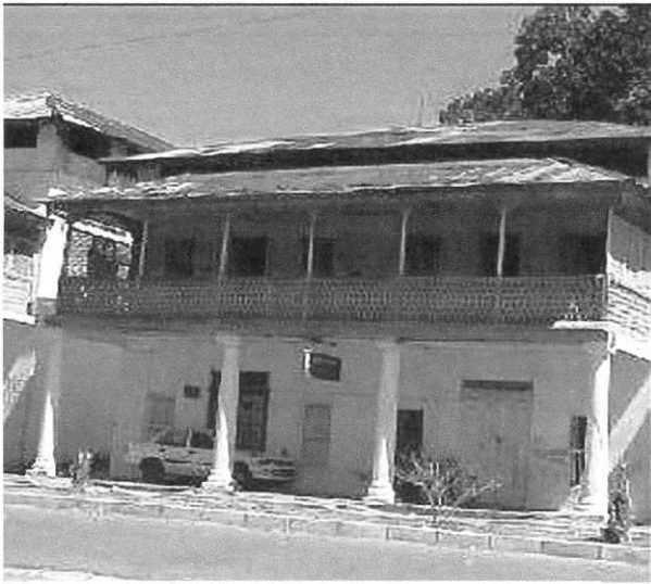
Plate 4.7: Persian Building with balcony and its roof was highly corroded due to high humidity and salt
