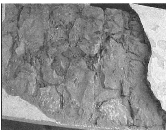
Plate 4.15;: Termites on the wall cause the peeling of wall plaster (Health building)
