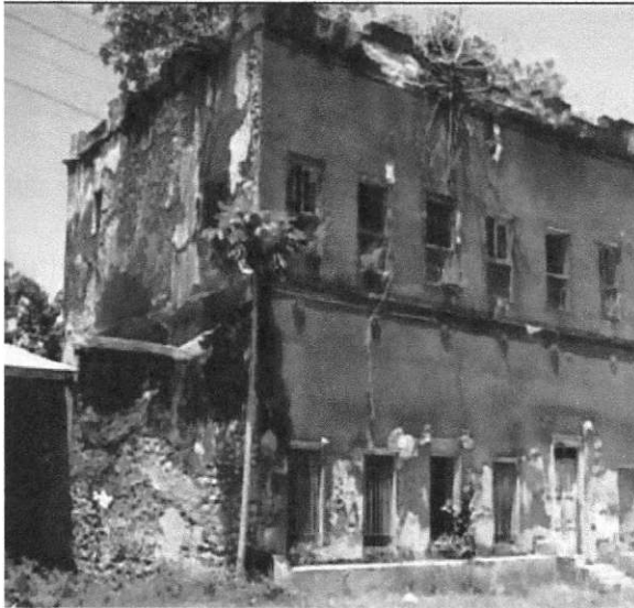
Plate 4.9: Slave building, PanganUPeeling off of walls, cracks and growth of vegetation due to climatic condition effects.
