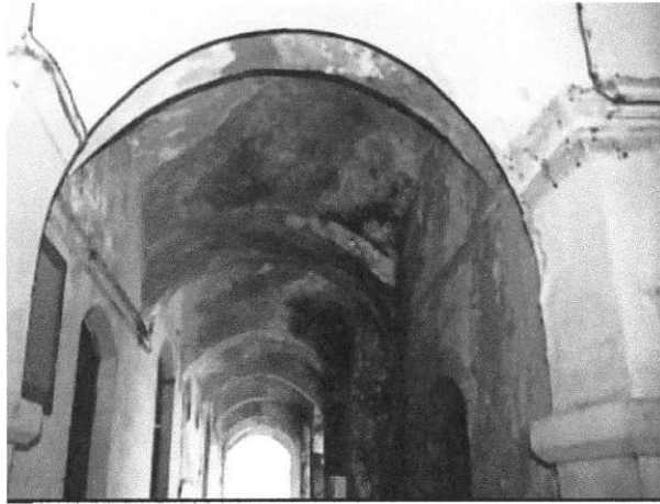
Plate 4.14; Peeling off of wall plaster inside the cliff block due to climatic conditions (Bombo hospital).
