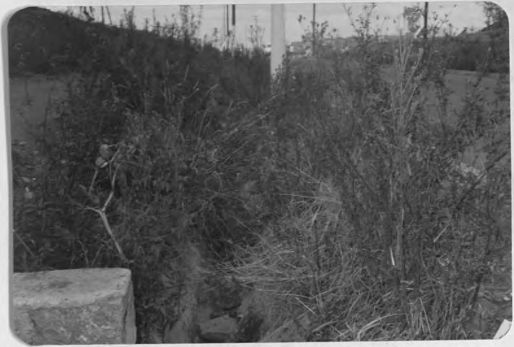
Plate 18: An open drain covered by a thick bush in Umoja II
