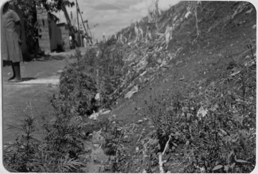
Plate 19: An open drain blocked by slumping earth mound in Umoja II.
