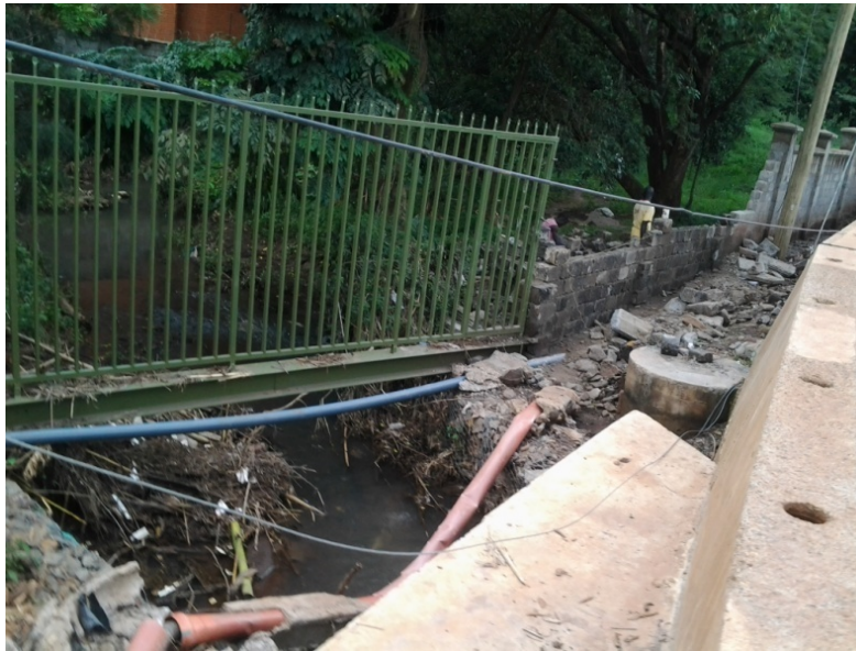
Plate 5.3 Boundary wall destroyed by flooded Kirichwa Ndogo river
