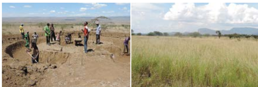
Plate 5 Community participate in digging soil and water conservation structures to control the Suswa gullies in Suswa and rehabilitation of degraded land through pasture re-seeding in Ewaso Ngiro, Narok.
