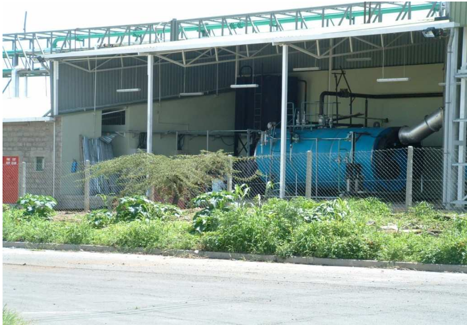
Plate 6 : A boiler at one of the enterprises
