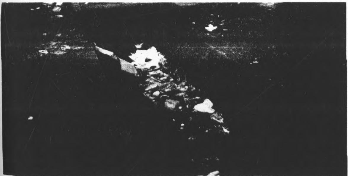
Plate 7: Blocking of open drains by solid waste
