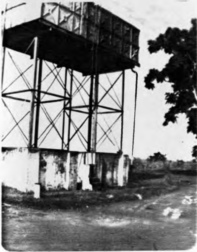
Plate 5 (a): The Water Reservoir. It is too small and is empty most of the time.
