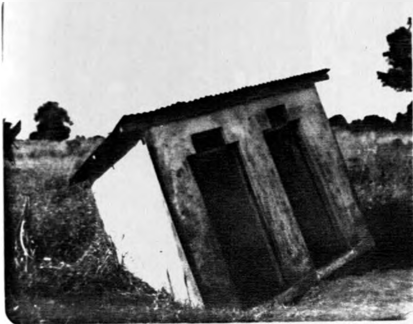
Plate 6(a): Latrines are few and poorly maintained.
