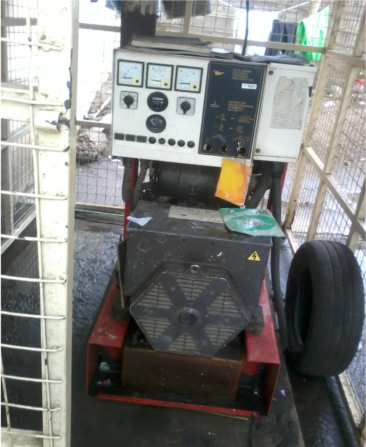
Figure 2.2 Nairobi West Petrol station Standby Generator Rating 30KVA 41.7Amp 3phase
