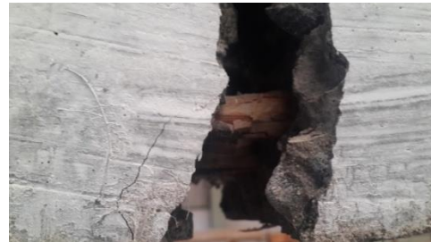
Figure 8: Slipped L.buchananii tensile reinforcement
