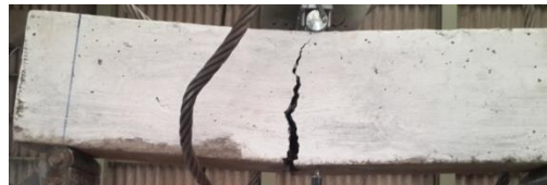
6.6: Failure pattern of L.B. 399
