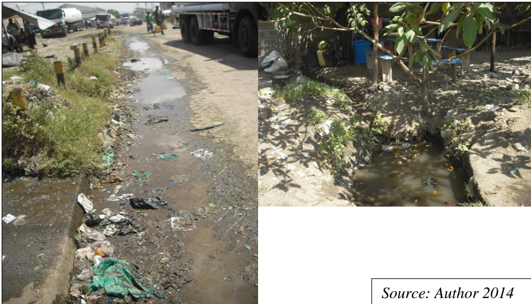
Plate 11: Drainage along Wundanyi road
